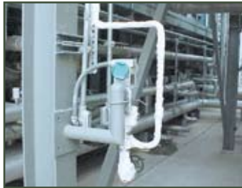
Typical Field Installations
